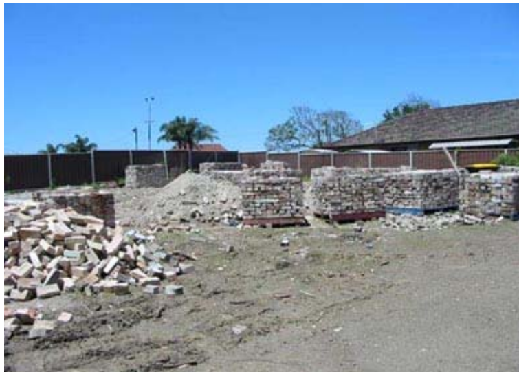
Example of recovery and recycling of bricks for re-use from a demolition site
