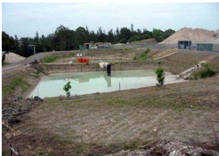
Site water management includes suitably sized sedimentation and detention basins, oil / water separators, turbidity and pH control, and capability to contain and recycle all waste water generated within the site.
